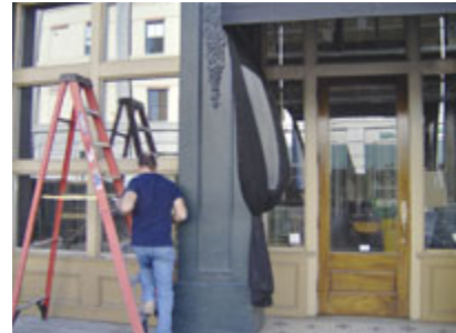
Work is underway at new site of Panera Bread at 1 West Broughton St., at the corner of Bull St.
